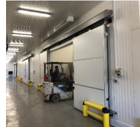
Turnkey Cold Stores
